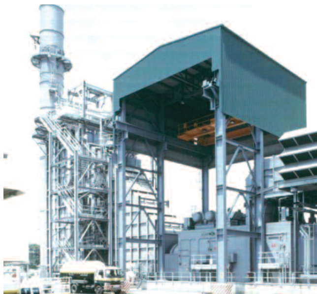
A 113 MW CHP plant sells power to EGAT, the state-owned utility (Bangkok Cogeneration)
