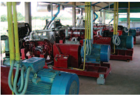
Modified truck engines and induction generators burn biogas to generate electricity at SPM farms (EPPO)
